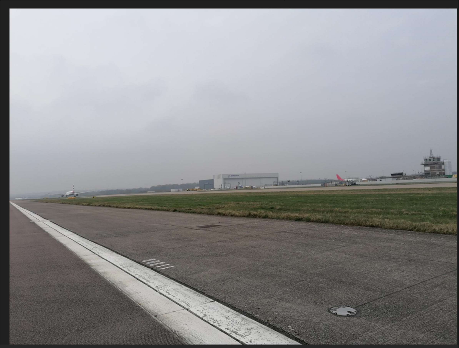
Appendix to Table 2: photograph (taken from the northern runway) showing the white line under which there is a drainage system.
